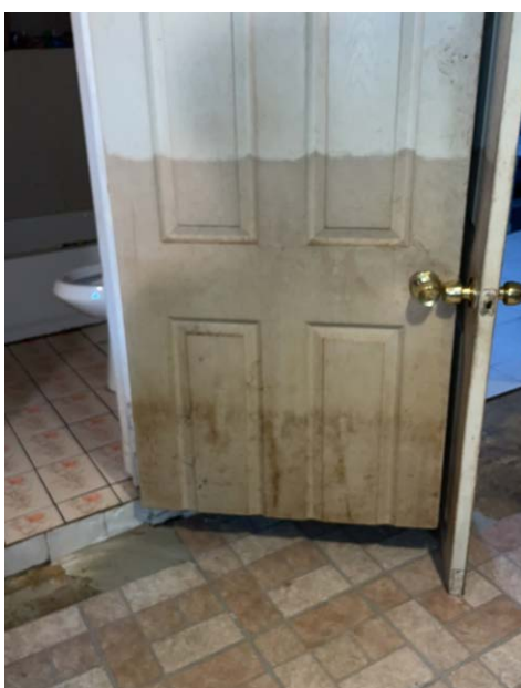
Figure 9: Flood Damage in Basement
